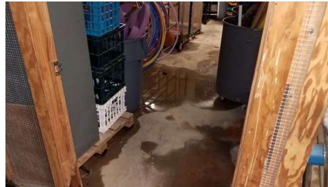
Above: the above picture shows a normal level of sitting water in the basement storage areas. Picture from 2021
