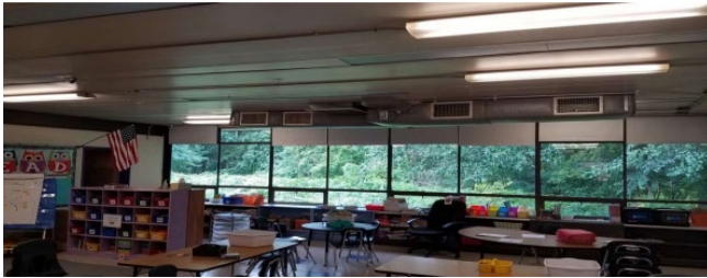
Above: the above picture shows loud and disruptive HVAC ductwork in the classwork. Picture from 2021 via Public Buildings.
