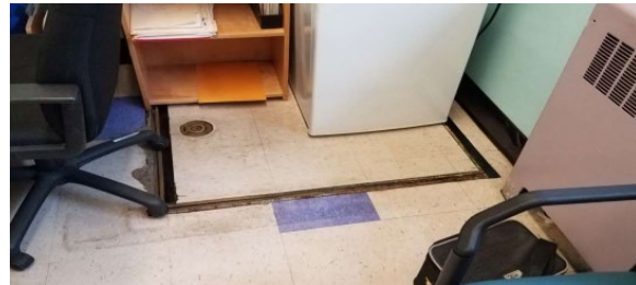
Above: the above picture shows the access to the sewage pump, which is located in the nurse's office. Picture from 2021 via Public Buildings.
