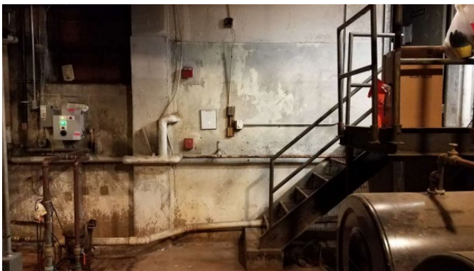
Above: the above picture shows damage 9 feet up on the wall from flooding. Picture from 2021 via Public Buildings.
