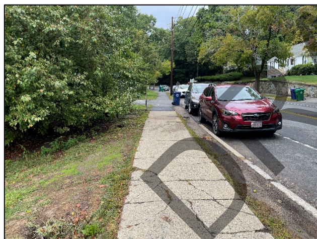
Photo 9: Instance of concrete sidewalk in poor condition beyond the intersection of Dedham Street at Walnut Street, along Walnut Street
