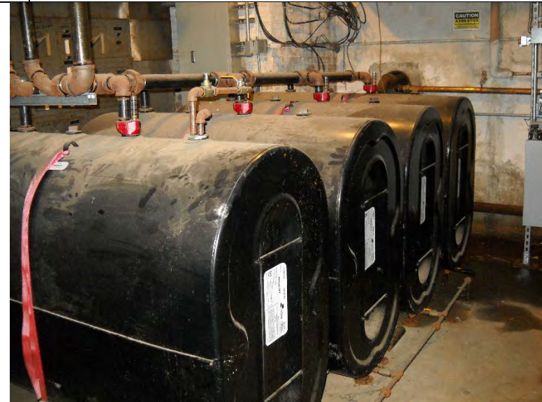
Photo #8: Four fuel oil ASTs in the boiler room.
