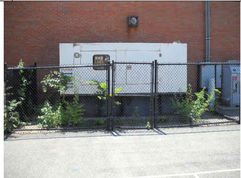
Photo #4: Generator and solar equipment at the north exterior of the building.
