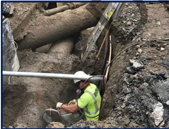
Water, Sewer, Stormwater Infrastructure
