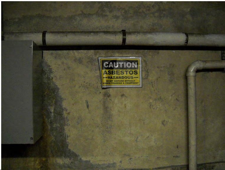
Photo #5: Asbestos placard in the boiler room at the Site.
