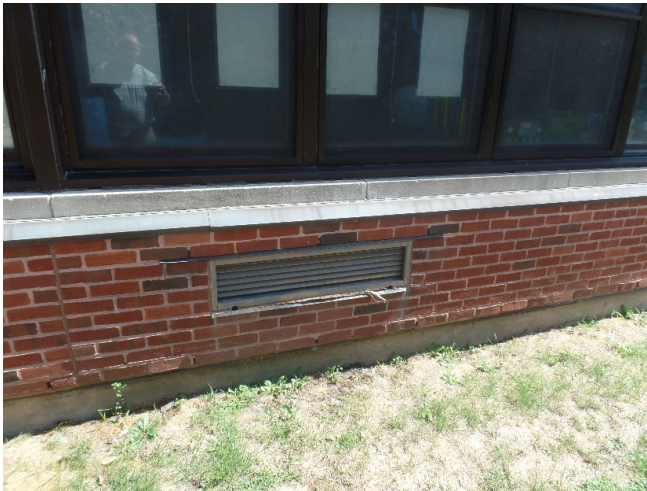
Photo No. 5: Unit ventilator grille at 1951 original building
