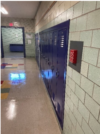
Pull station not at door
