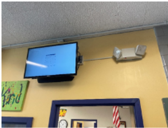
Emergency battery units
