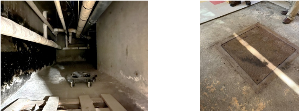
L - Pipe space runs along the perimeter to feed the radiators and unit ventilators. R - One of the many access panels to the pipe space
