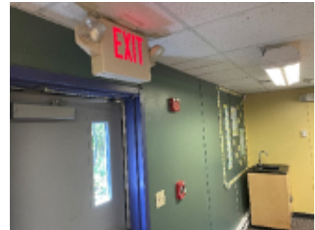
FA devices, emerg. lighting / exit sign
