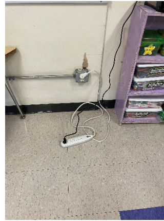
Power strip / Receptacle
