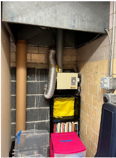
Kiln hood and exhaust are no longer used.
