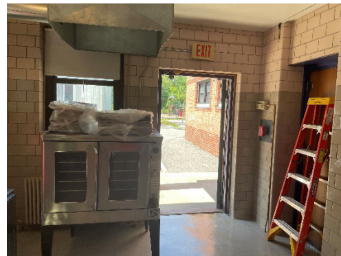
Exit sign not working
