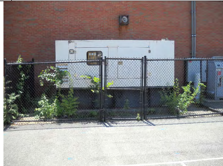
Photo #4: Generator and solar equipment at the north exterior of the building.
