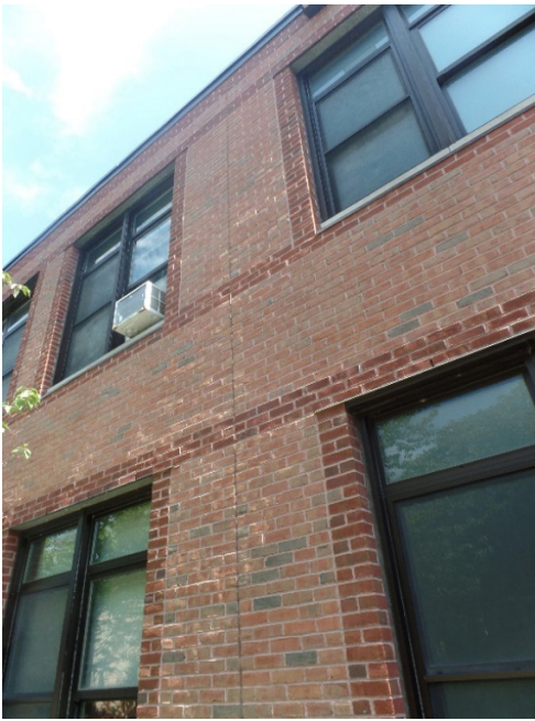
Photo No. 3: Standing water in 1951 basement
