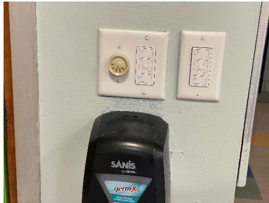
Typical room lighting controls
