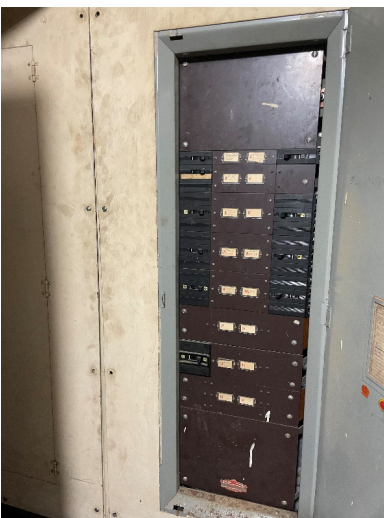
Original 1953 distribution panel
