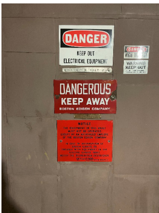
Transformer vault door. Need to confirm transformers have been removed.
