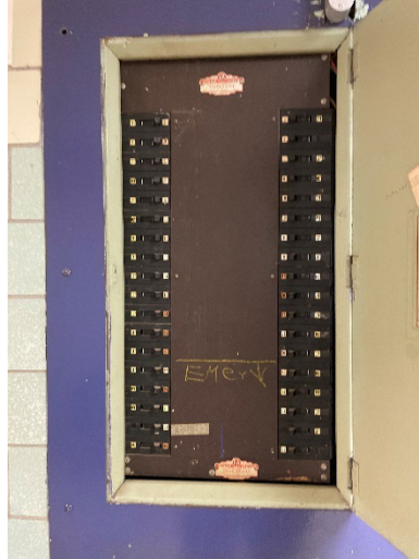
Panel in corridor
