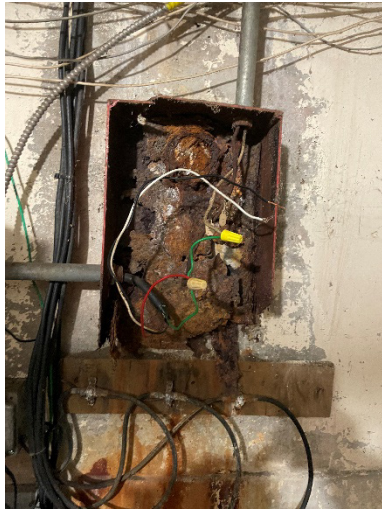
Water damaged equipment
