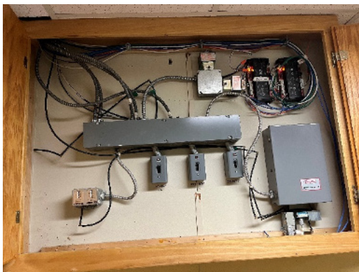
Delta DDC Controllers were found in the modular building.
