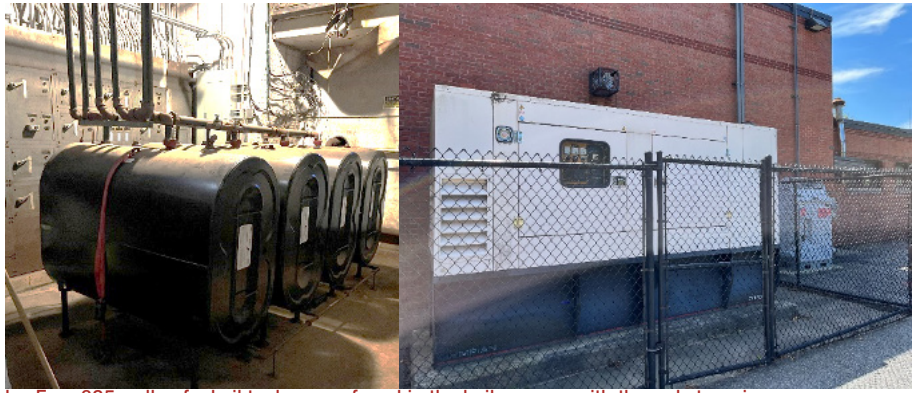
L - Four 325-gallon fuel oil tanks were found in the boiler room, with the red strapping apparently installed to prevent floating during floods. R - Diesel standby generator with a belly tank.
