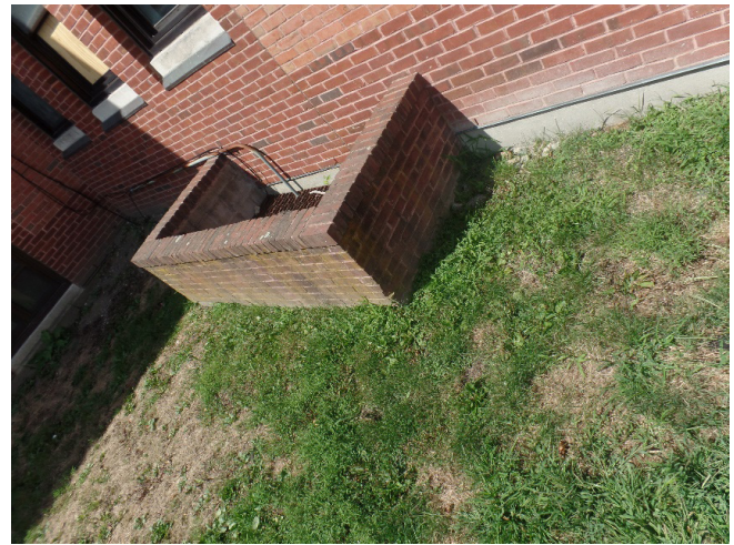
Photo No. 6: Brick deterioration at 1951 building areaway walls
