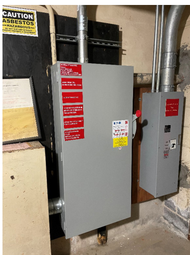
Service #2 and PV disconnect switch
