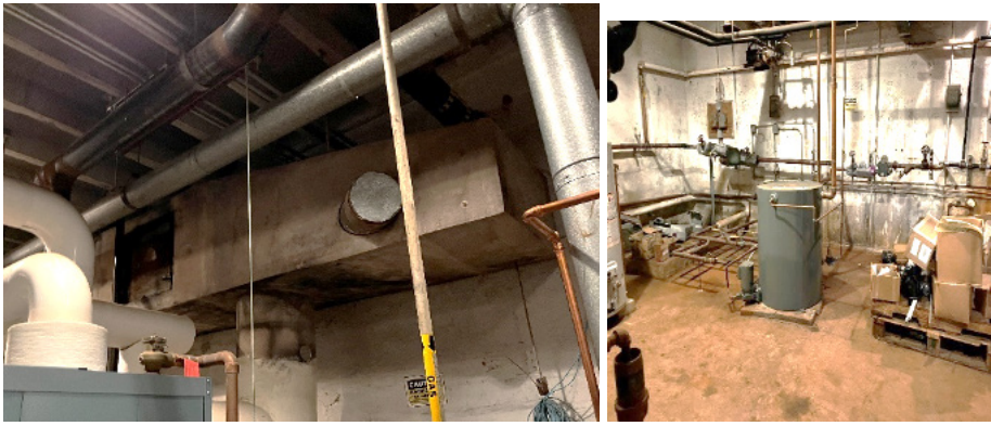
L - Original vintage boiler breeching. R - Recently replaced condensate receiver, but all the piping are the original. Note that entire floor is deeply stained from chronic flooding.
