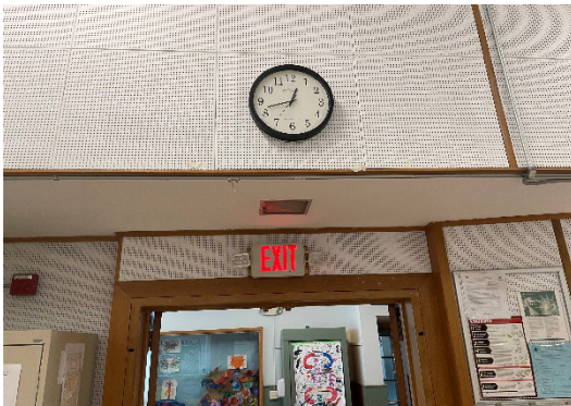
Exit sign with emergency lighting
