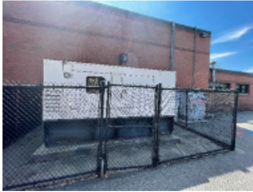
Generator with PV equipment adjacent
