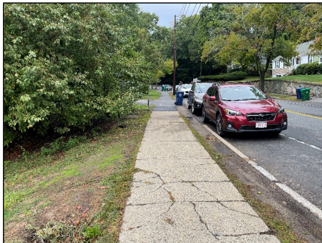
Photo 9: Instance of concrete sidewalk in poor condition beyond the intersection of Dedham Street at Walnut Street, along Walnut Street
