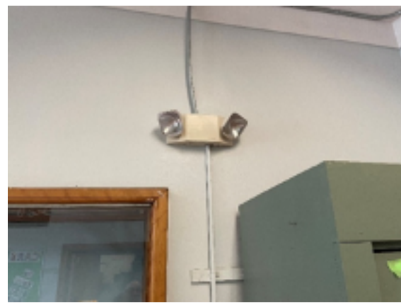
Emergency battery units
