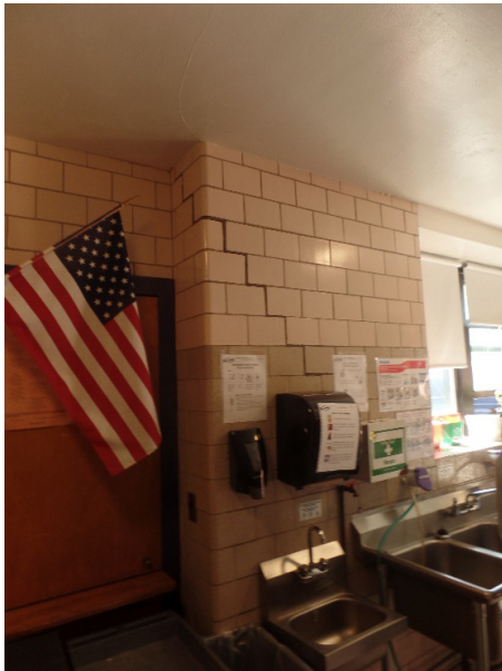
Photo No. 9: Step cracking in masonry in 1951 building
