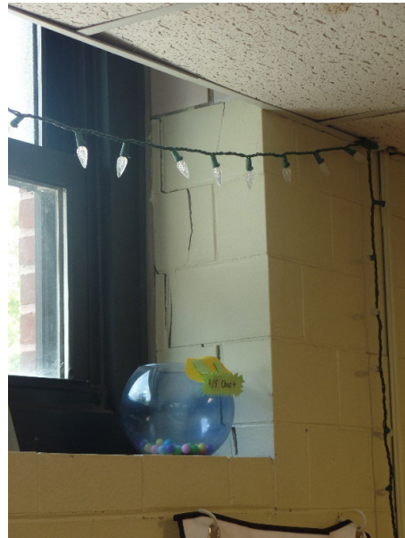
Photo No. 10: Cracked masonry at 1951 west wall window jamb
